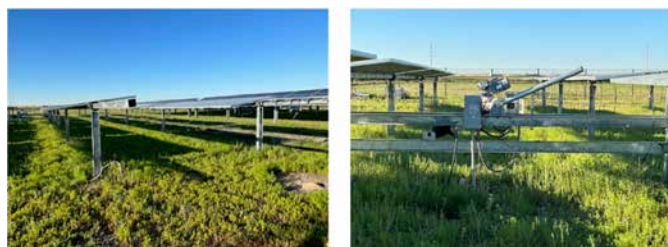
EPRI's outdoor test facility near Denver, Colorado, showing dedicated tracker rows to be used for field studies.
